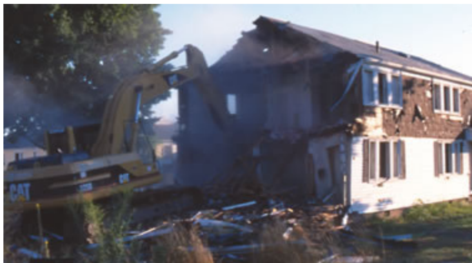
The demolition of Long River Village during the summer of 1999. Many residents came to watch and pick up mementos of their former homes. Photo by Nancy O. Albert from a project commissioned by the Middletown Housing Authority.
